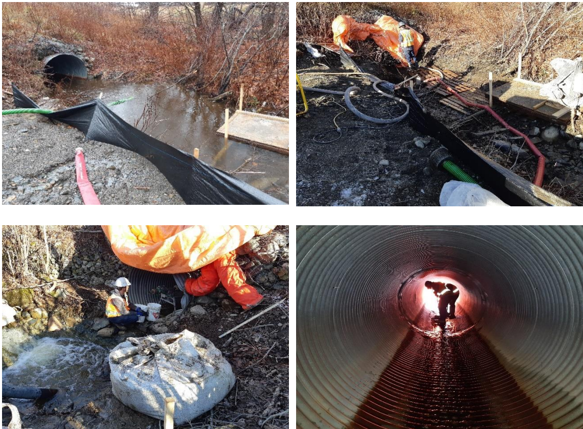
Figure 3.4. Southern side of CSP before pumping (top left), Southern side of CSP after pumping (top right), northern entrance of CSP during pumping (bottom left) and stopped flow culvert and cleaning process (bottom right).
