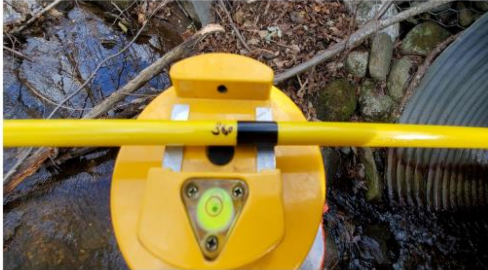
Picture 10. Tripod near the inlet of the CSP as a reference for incrementing the LIDAR between full scans. Marking along the fibre glass pull rod to make Z axis locations.
