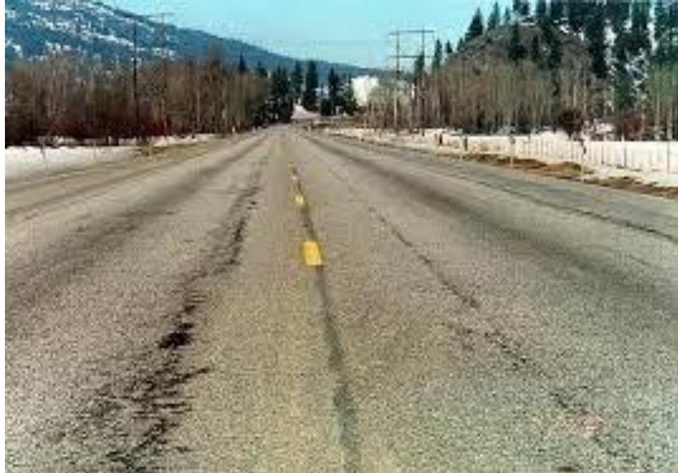
Figure 2.7 Raveling on the Surface of Pavement
