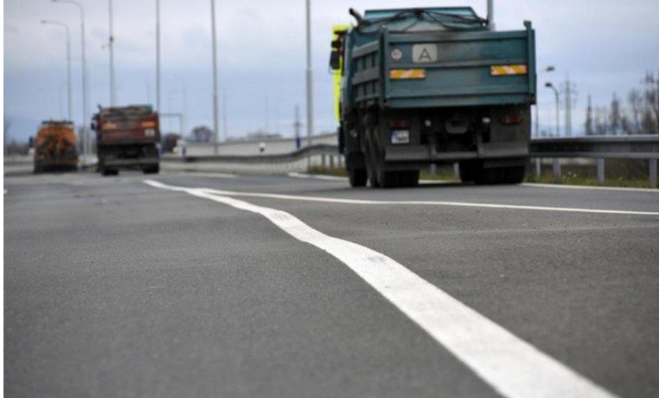
Figure 2.12 Settlement on Pavement Surface
