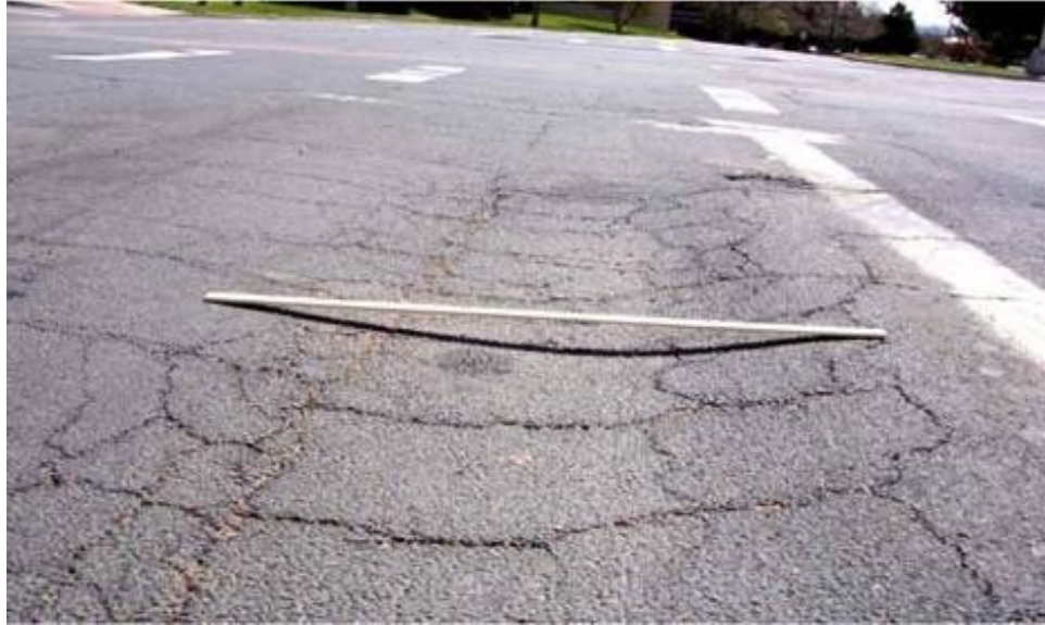
Figure 2.9 Rutting on Pavement
