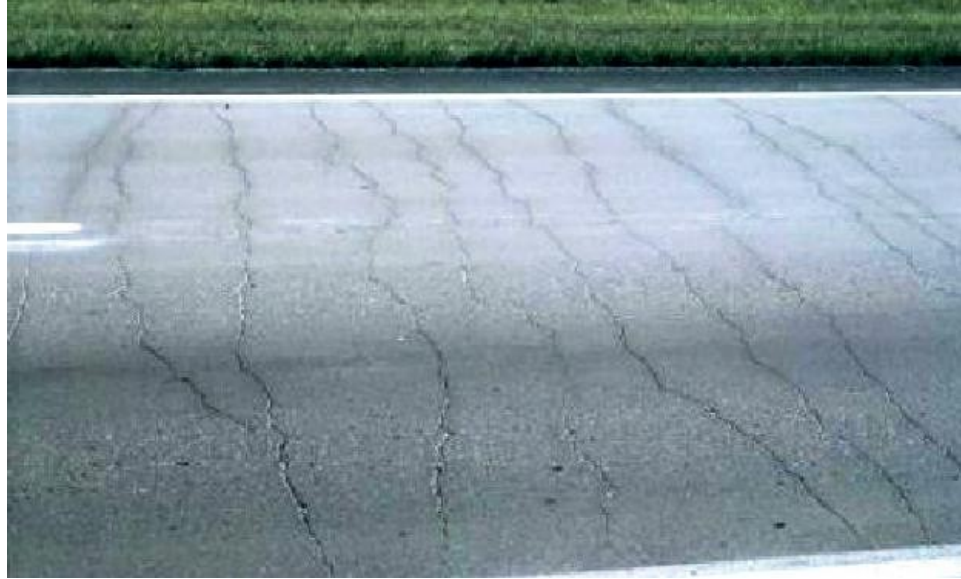
Figure 2.8 Thermal Cracking on Airports Pavement
