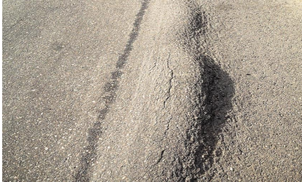
Figure 2.11 Shoving in Pavement
