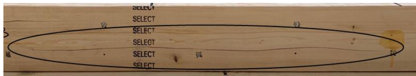
Figure 44 Extensive internal splitting in lumber (No. 74), specimen 3-2-H
