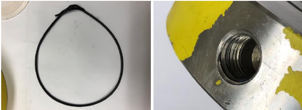
Figure 4.6: Faulty O-ring and thread from loop II pump
