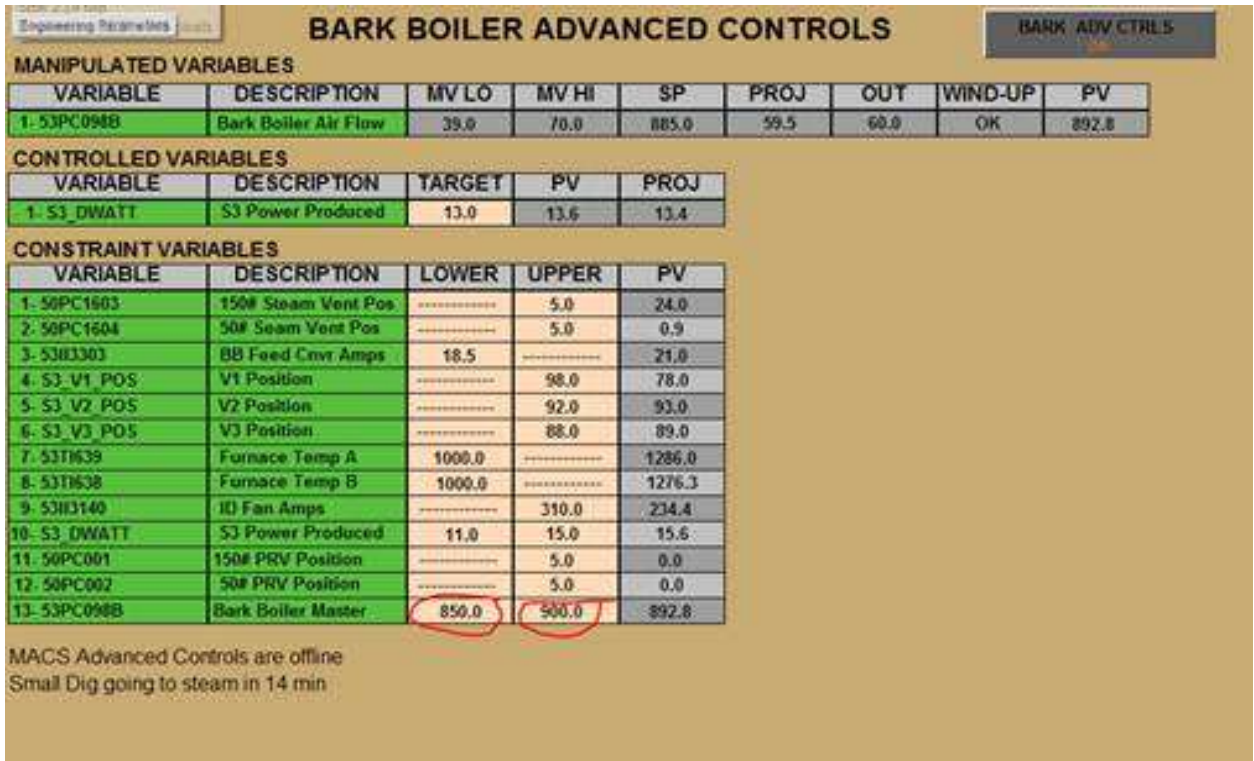
Figure 3.29 Multivariable Advanced Control DCS Interface
