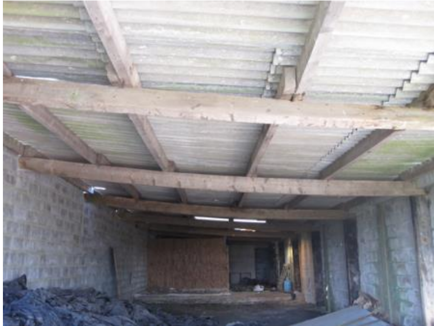
Figure 1.7 The bent roof beam because of long-term loading. (Source: https://www.iom3.org/wood-technology-society/creep )
