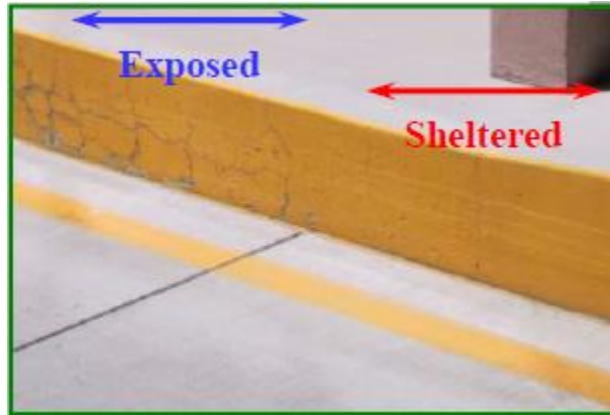
Figure 2.15: Damage difference of concrete exposed to and sheltered from moisture (Thomas, 2016a)
